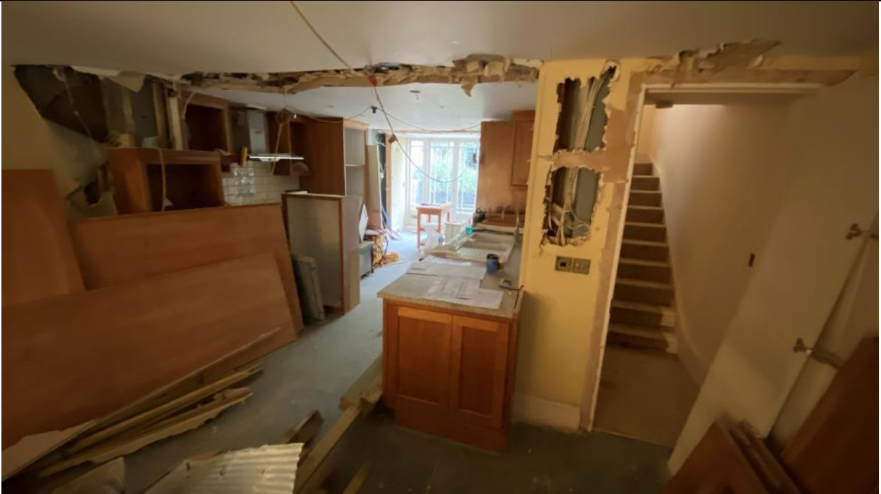
Photo 3: Lower Ground Floor - looking from front to back including staircase proposed to be replaced.
