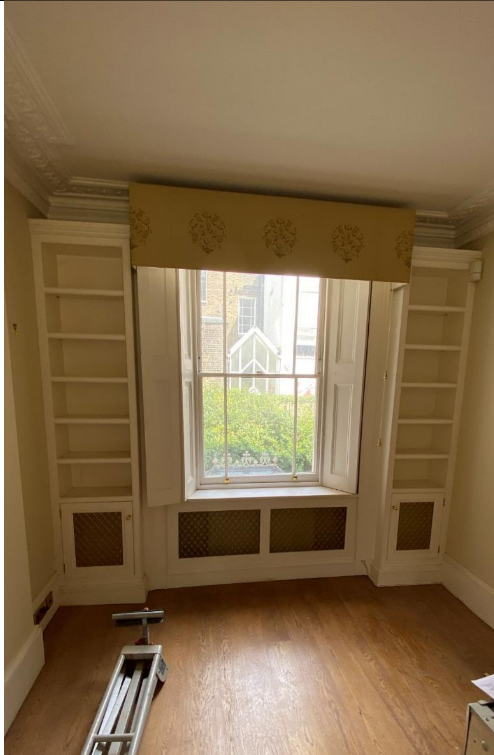
Photo 4: Ground Floor - View of rear window proposed to be converted to French doors onto balcony
